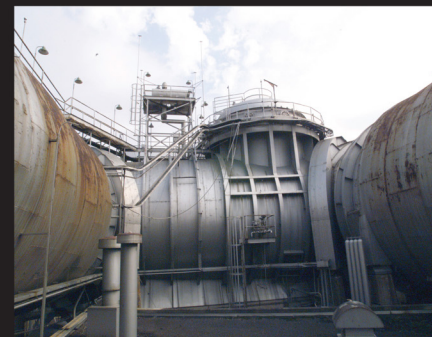
Space Power Chambers' vacuum tank with removable dome was located near the southeast corner of the former AWT. In 1961 and 62 the AWT was converted into two test chambers. After the acquisition of the Centaur Program in October 1962, it was decided to add this dome to the space tank so that a Centaur rocket could be stood up vertically inside. The addition of the dome delayed the use of the facility for nearly a year.
