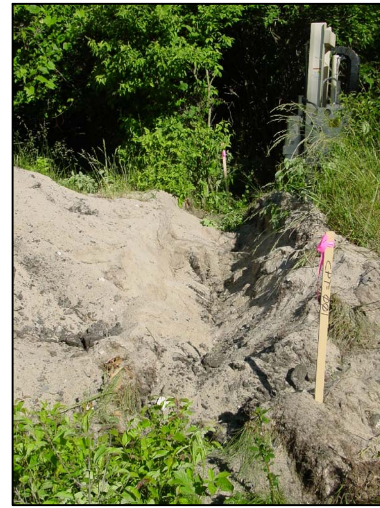
PHOTO 4 (CDP Trench Through Spent Sand Blasting Grit at FR-5)
