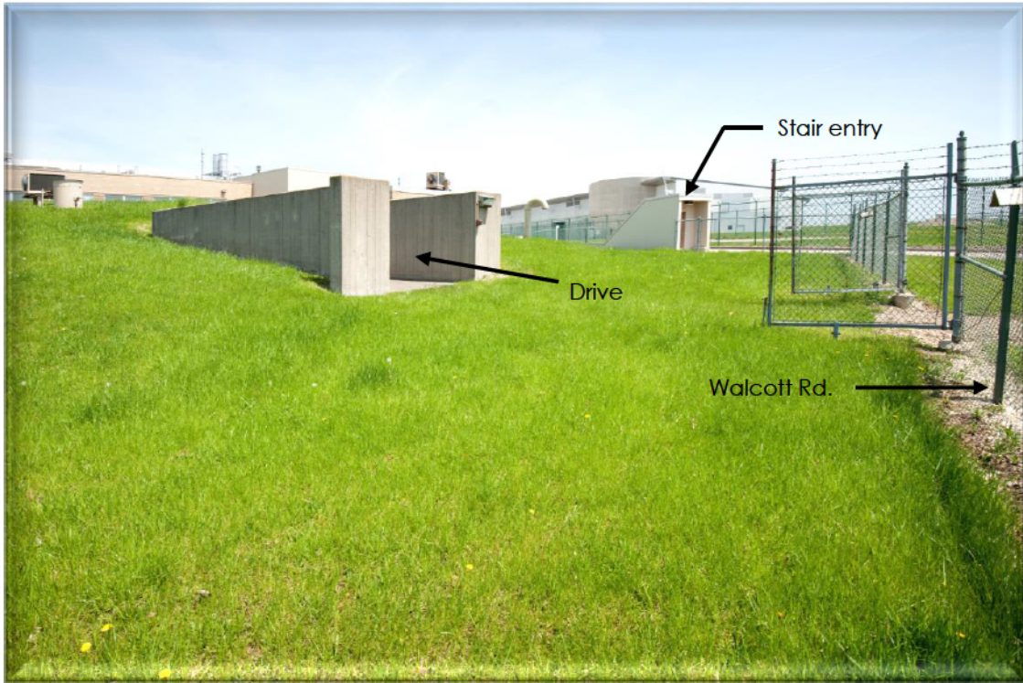
Entry into drive to above ground Mechanical Room from Walcott Road Photo 1
