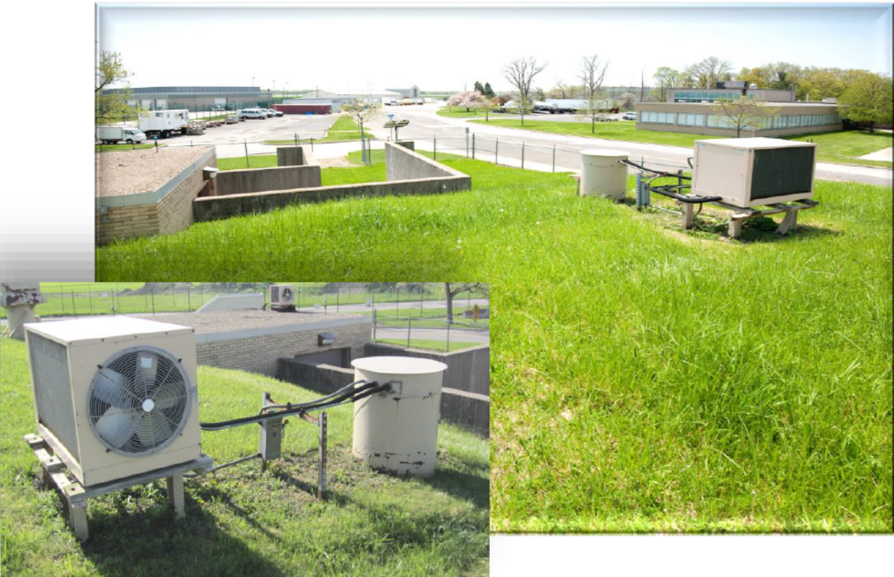
View of A/C Condenser Unit Photo 4
