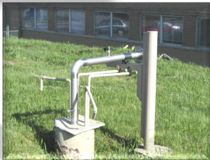
Abandoned Utility Lines Photo 11
