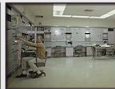
B-3 Control Room
