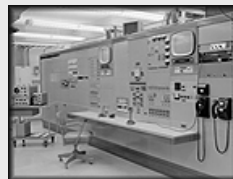
B-1 Control Room
